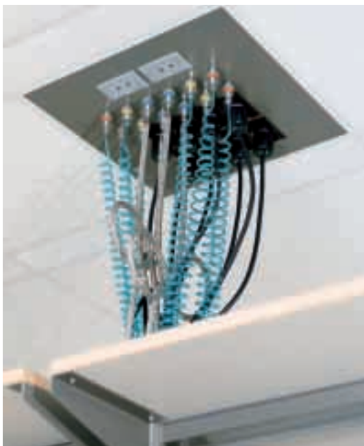
All service lines are innovatively piped and wired for quick connection to the movable ceiling service panel.
